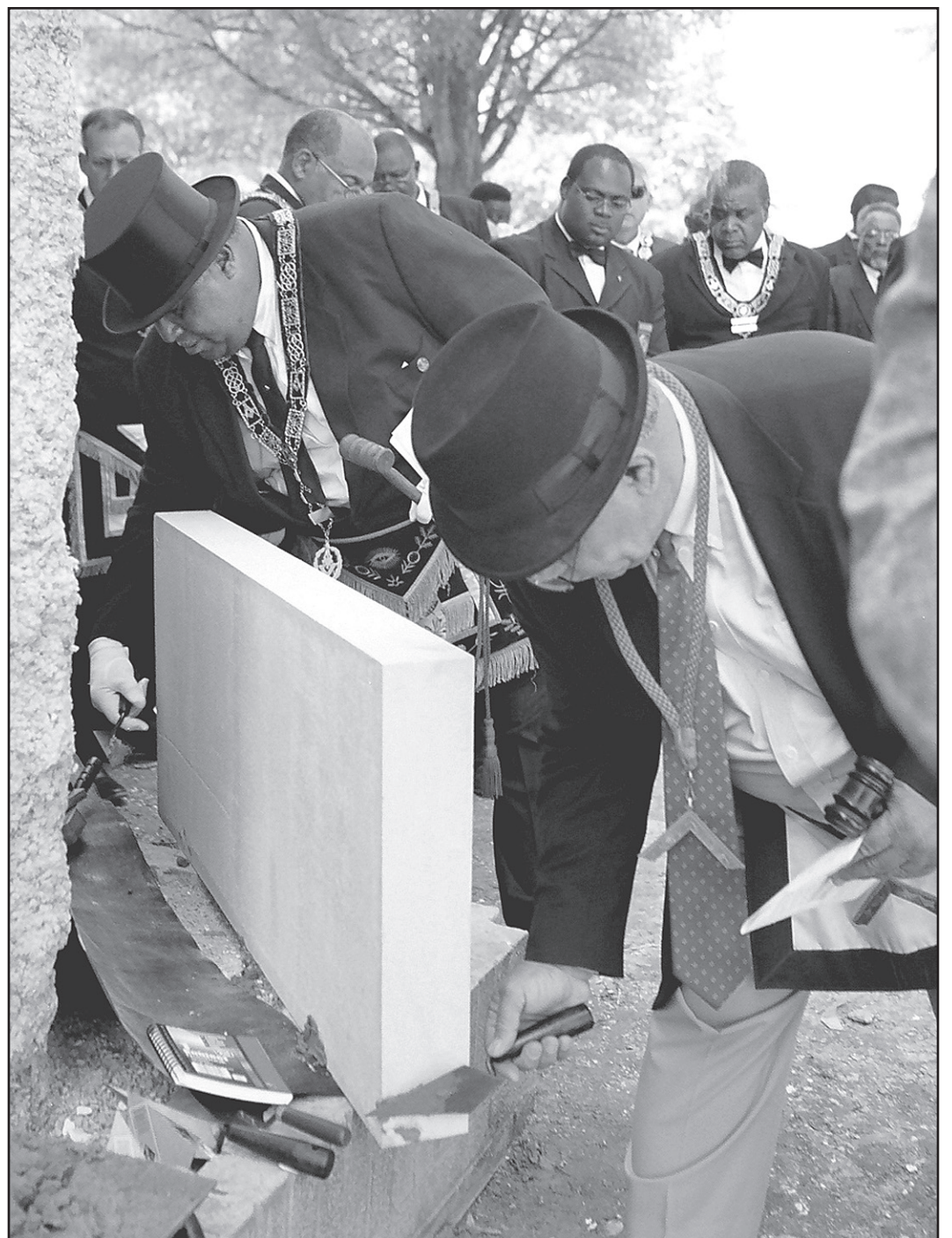
Grand Master stand-ins James Alford and James Chavis spread mortar on the cornerstone of the new Richmond County Courthouse, above. At left, Grand Masters Rice and Fitch enjoy their joint appearance and the production of the first cornerstone with two GMs.
