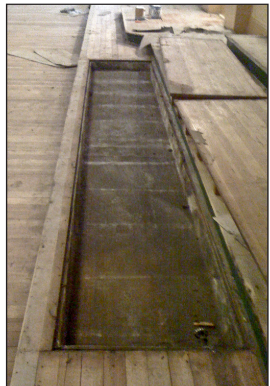
The positioning of the sink under the concealing floor is seen here.
