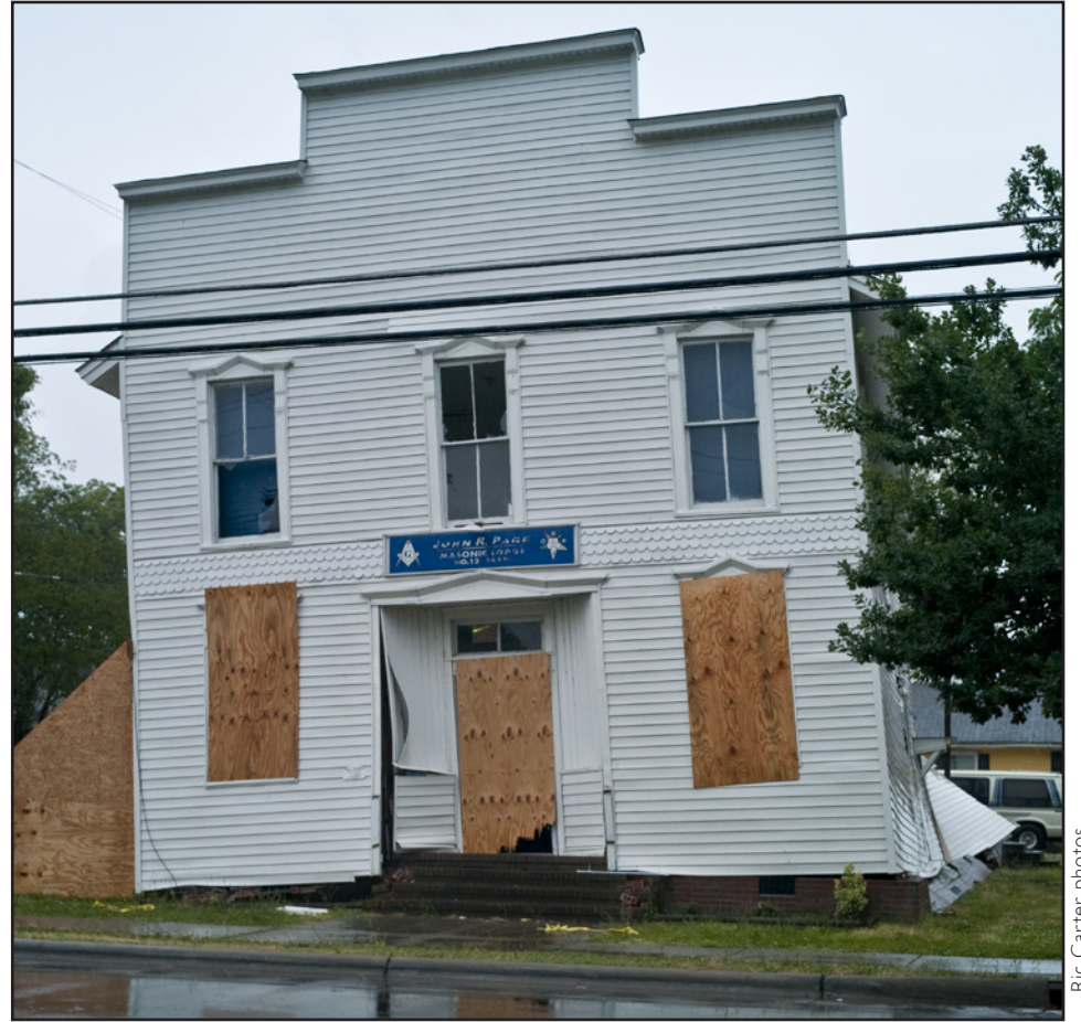
John R. Page 13 PHA suffered dire damage when blown off its foundation in an April 9 storm. They are just four blocks from Unanimity 7.
