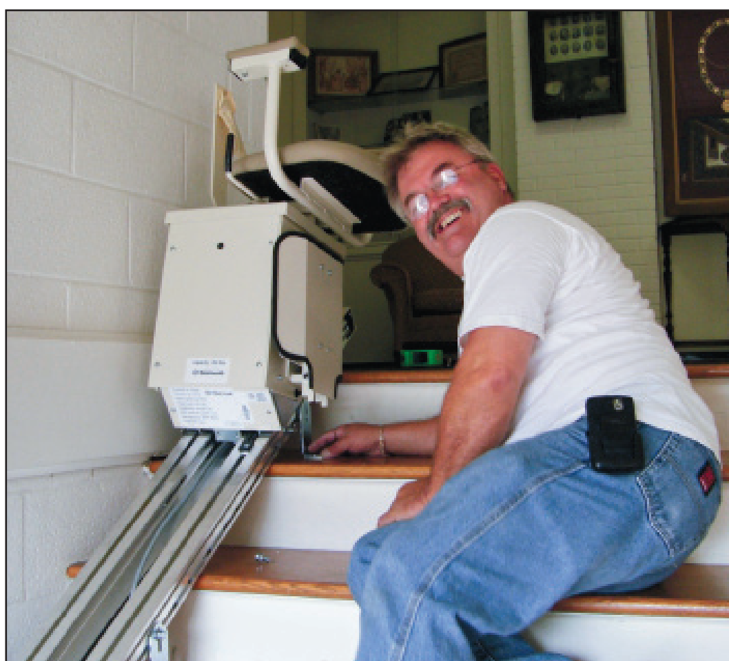
2010 Master Harvey Ellis is seen here installing one of the lift chairs.
