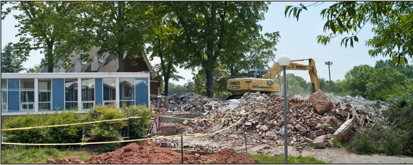
The landscape by the chapel at WhiteStone is changing drastically as construction nears.
