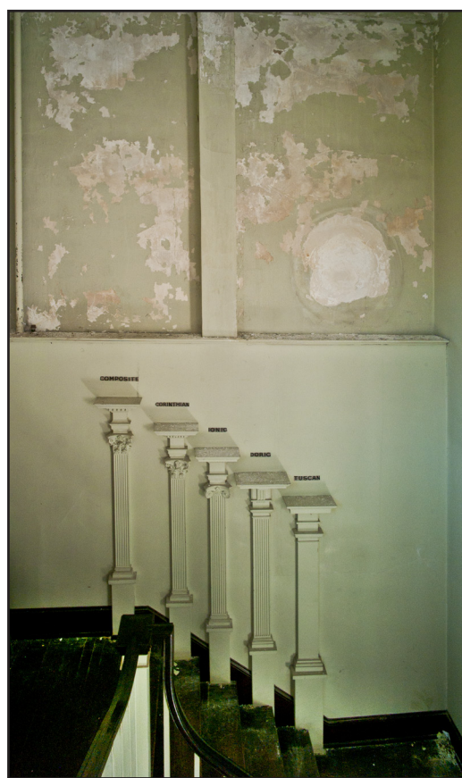
Greensboro Masonic Temple's winding stair goes from flaking to spit shine.
